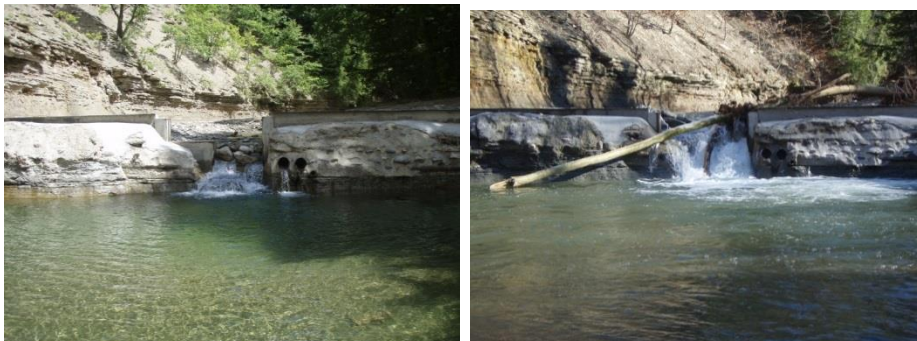
Figure 2c-3. Notching in the lower dam post-construction and pre-flood, and logs and rocks in notch after the Superstorm Sandy flood.
